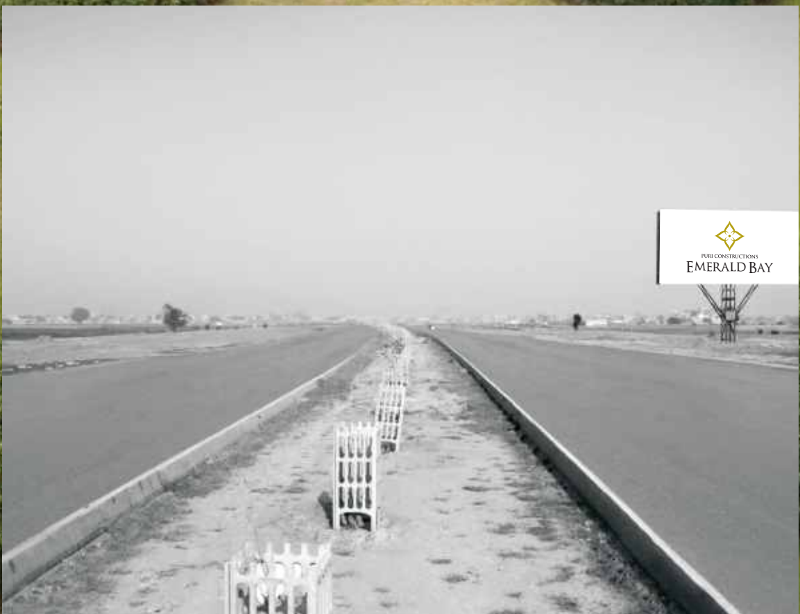
Actual picture of Dwarka Exressway under construction right at the frontage of Emerald Bay.
